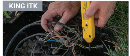
42025 - Irrigation Tester Kit with Tone Probe Irrigation tester plus Tone Probe to ID individual wires
